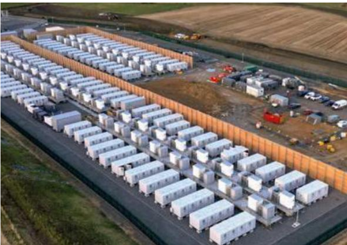
Grid-scale energy storage system
